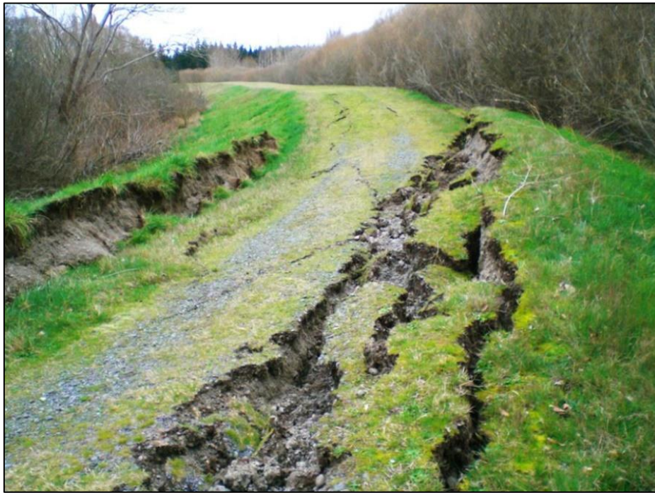
Figure 2-9 – Example of an earthquake damaged stopbank after the 2010 and 2011 Darfield and Christchurch events (Bainbridge, 2013).
