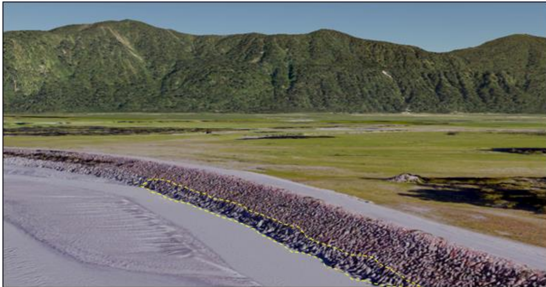
Figure 3-12 – A slumped section (yellow dashed lined) of the Milton's stopbank.
