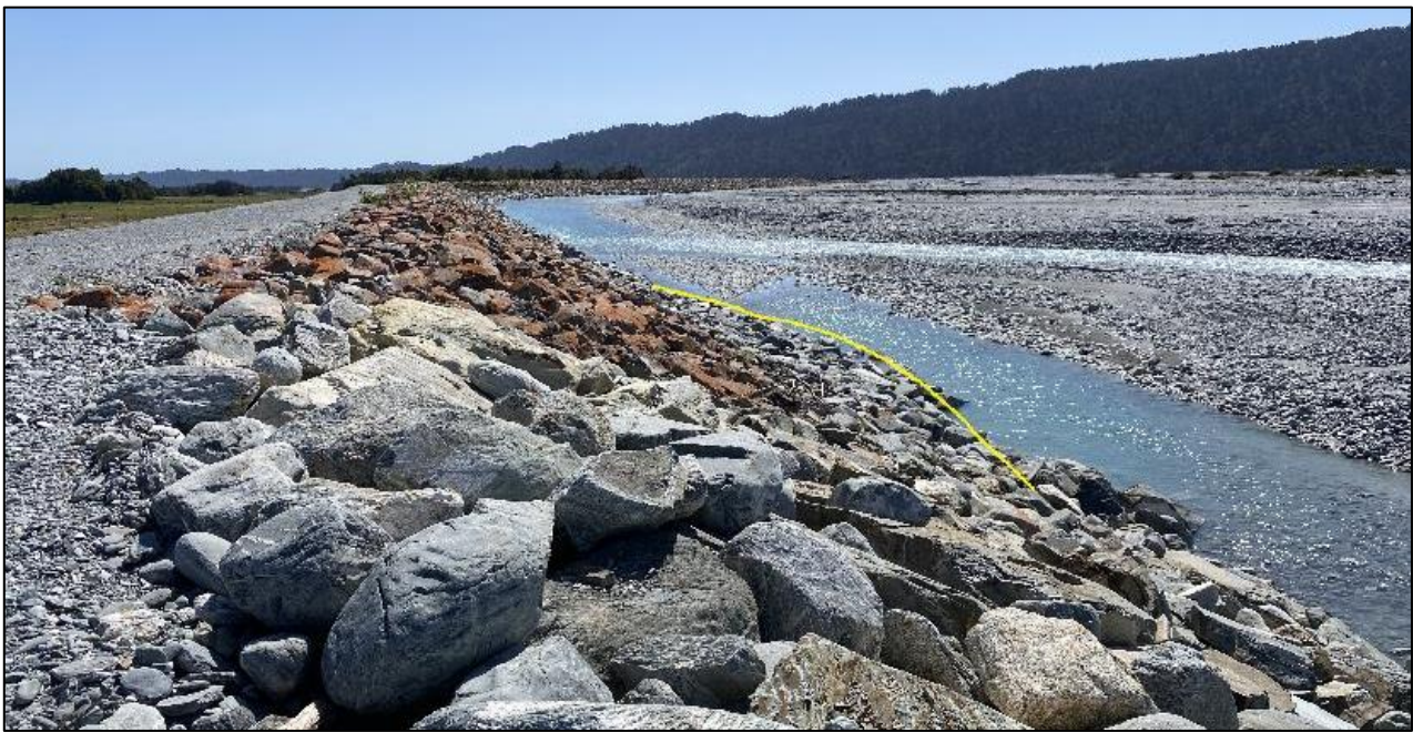
Figure 3-11 – A section of slumped rock on the Milton's stopbank , as shown by the yellow line.
